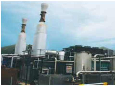
The gas engine drives a turbine
